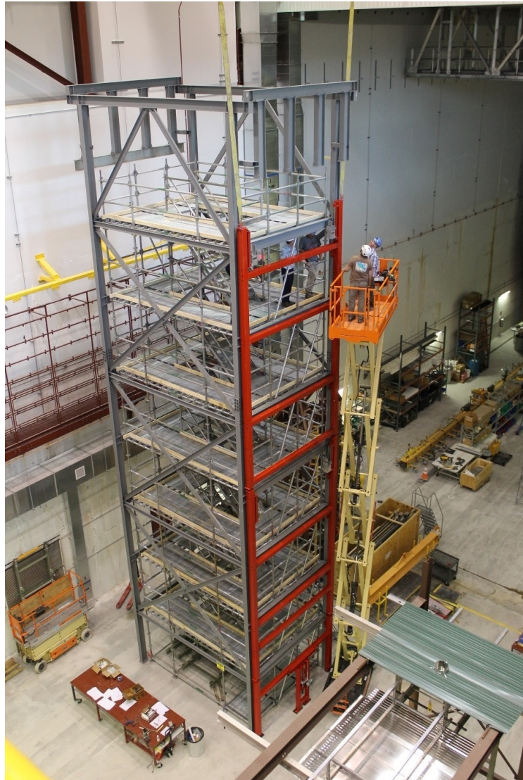
Figure 4.6. Phase 1 APA installation frame (in red) being installed on the APA assembly tower at Ash River. In the foreground is the ProtoDUNE-SP trial assembly structure.
